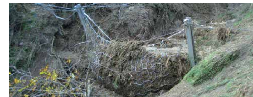
Debris Flow Barrier
