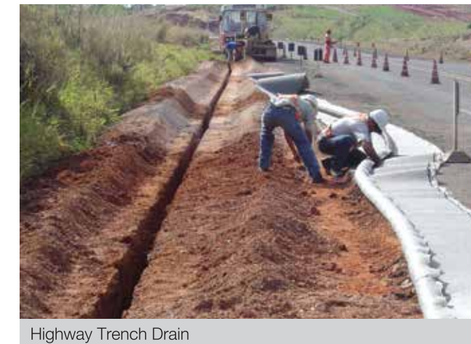
Highway Trench Drain
